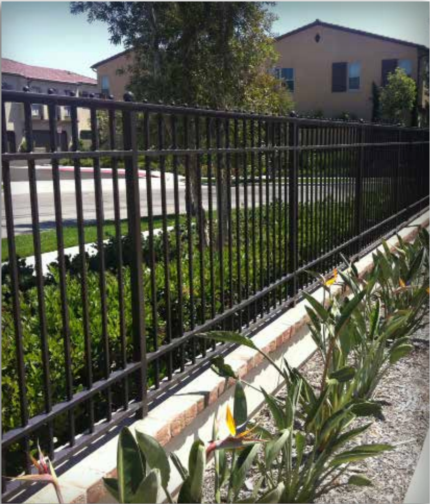
Tubular steel fencing
